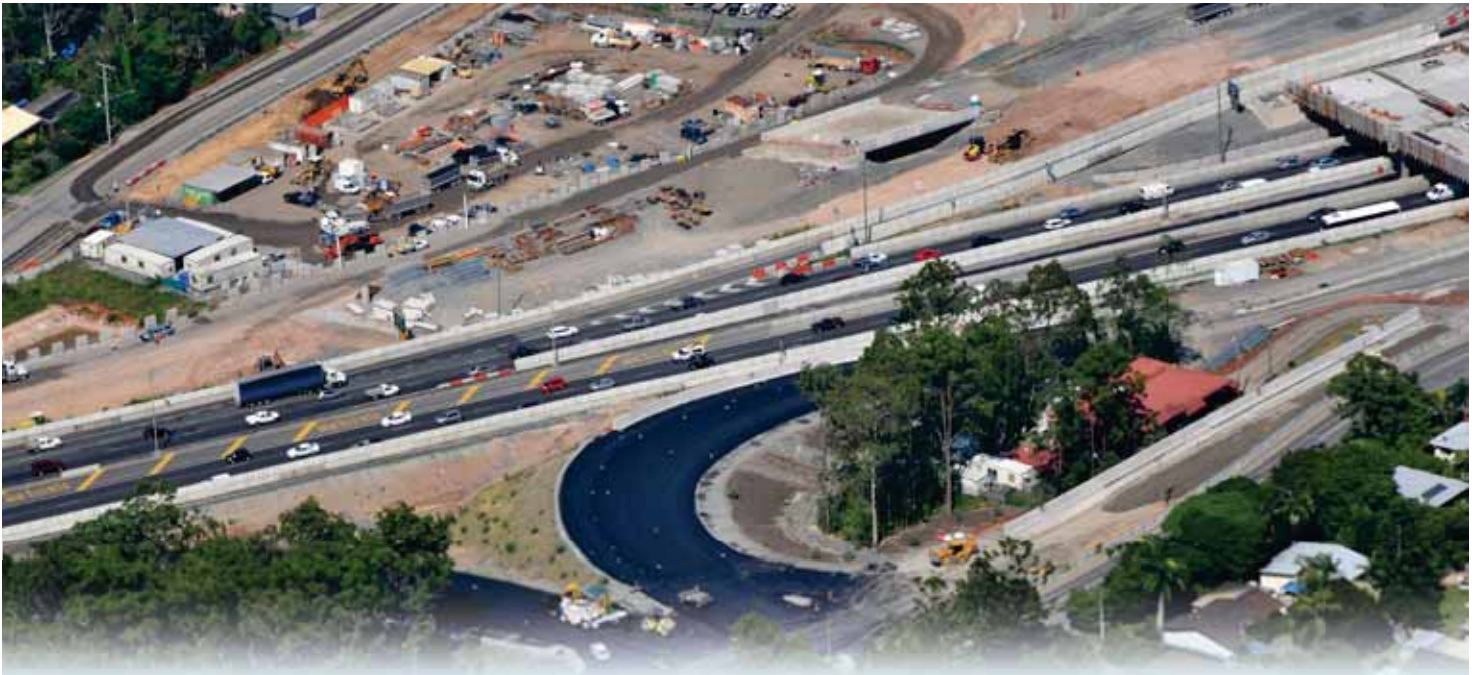
Works are progressing to construct the new southbound Winnetts Road on and off-ramps and northbound Loganlea Road off-ramp.
